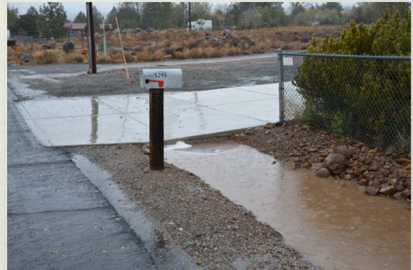
Photograph taken on October 16th, 2016 at 5:26 PM of 12" culvert on Shawna Lane. Note that discharge is at capacity for this storm water system.
